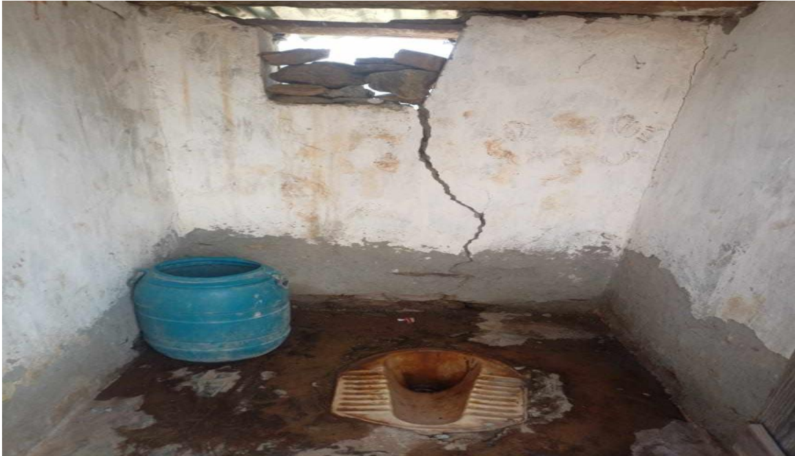
Figure 5 Dysfunctional Household Toilet
