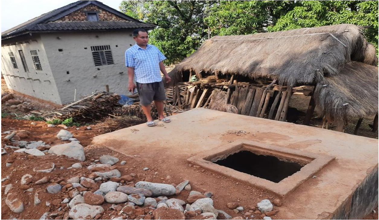
Figure 10 Useless of Reservoir Tank (RVT)
