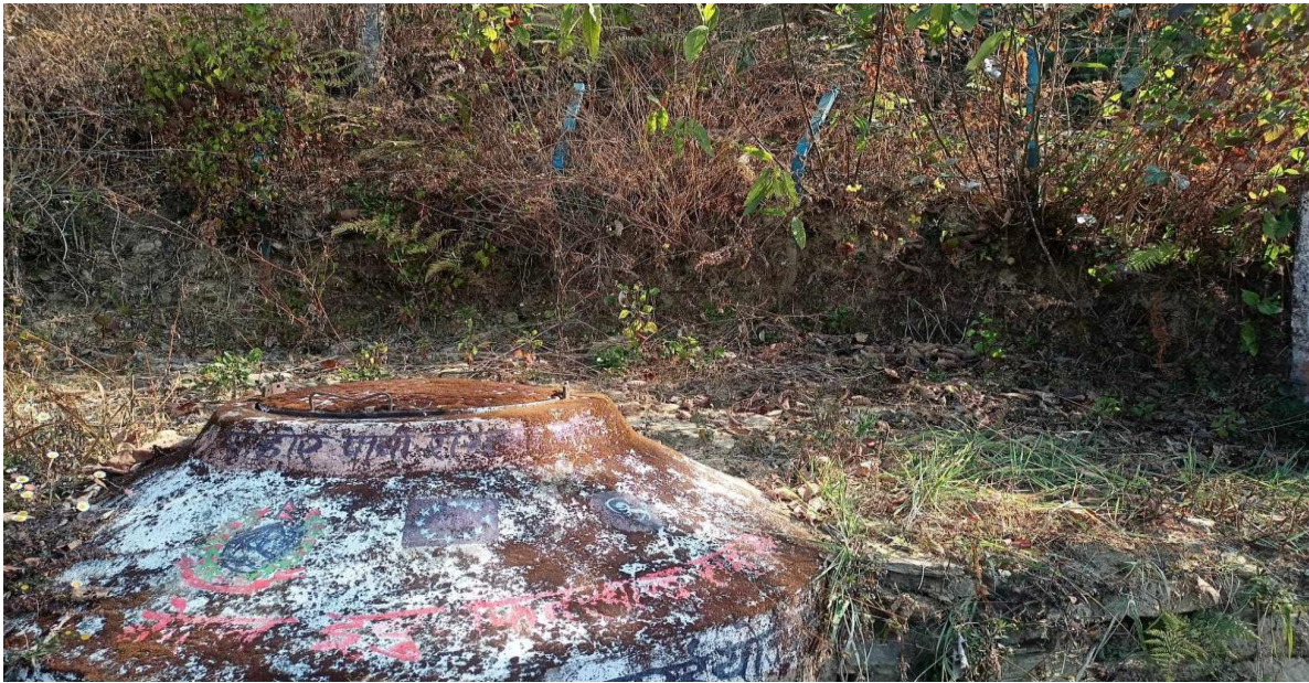
Figure 2 Non-Functional Water Structure
