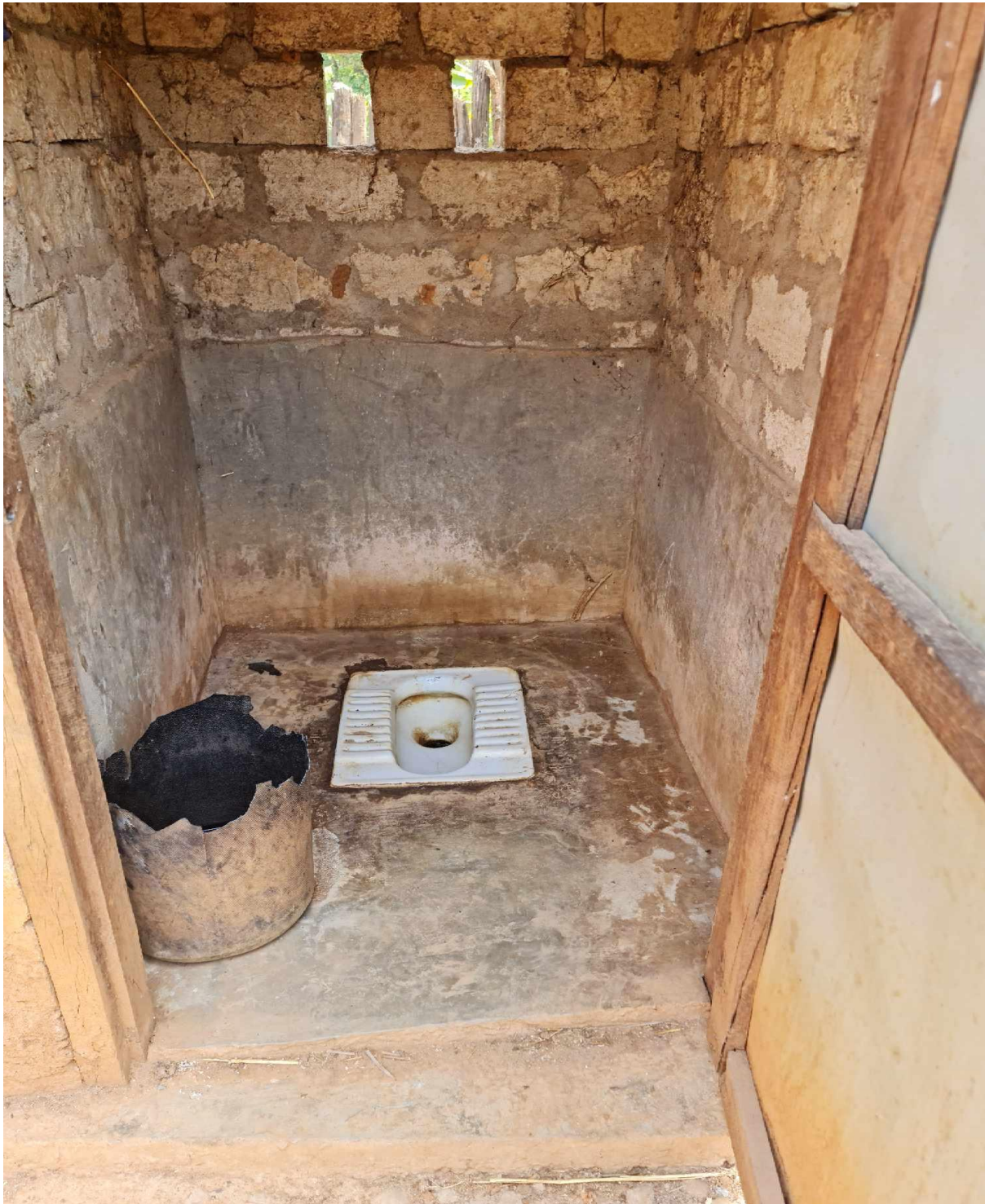
Figure 15 Toilet constructed but out of use due to water scarcity
